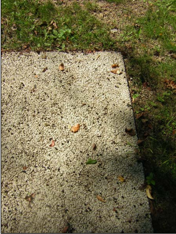
Figure 22: Surface Condition, Fred Fuller Park
