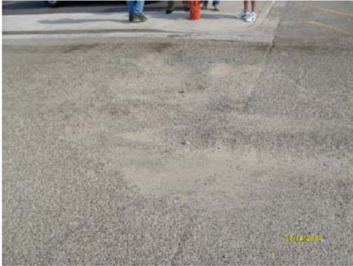
Figure 9: Surface damage from heavy vehicles near fire hydrant
