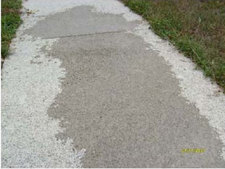
Figure 5: Sheet flow across clogged surface (observed at Rieth Village, Albion, Indiana)
